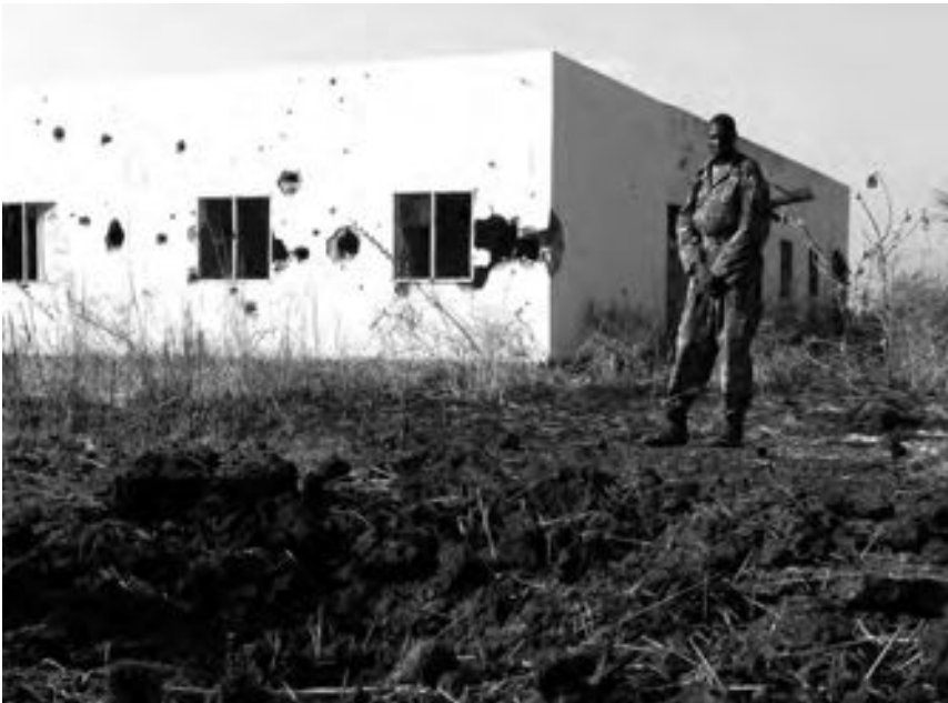
Image 5: Effects of the aerial bombardment conducted over Chali al Fil on 29 November 2012 on the local health care centre, built in 2008. Bombs also fell in the immediate vicinity of the mosque, setting fire to the building.
