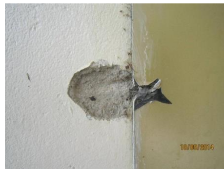
Fig 12: Bullet defect at edge of shown on the left
