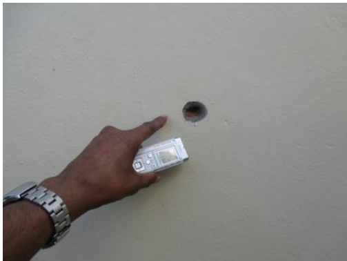
Fig 19: Bullet hole in wall of surgical theatre
